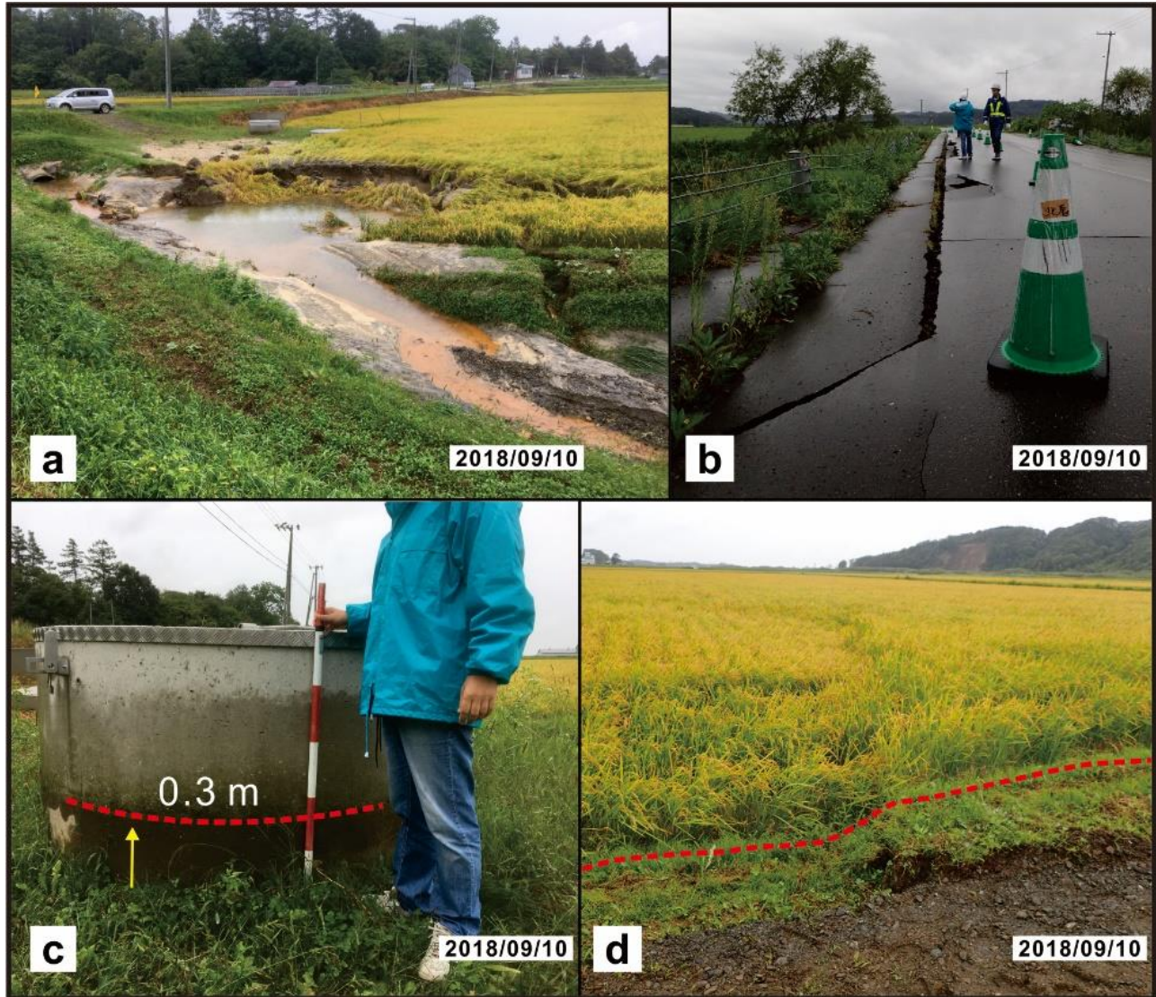
Fig. 5.3 Damages and liquefactions resulted from the Iburi earthquake sequence. (a) Liquefaction and jetted sand in the paddy field. (b) Road damage. (c) Uplift of inlet well. (d) Surface rupture in the paddy field
