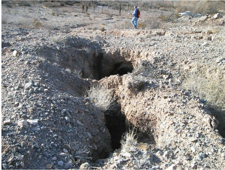
Figure 2.2 Formation of jugholes in an auxiliary spillway of Diablo Arroyo Site 1, Hudspeth County, in the Trans-Pecos area of Chihuahua desert, USA (Image source: USDA NEH 633.13 )
