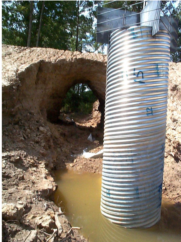
Figure 2.1 The 2002 piping failure of the Lonesome Dove Reservoir levee in Louisiana, USA (Image source: USDA NEH 633.13 )
