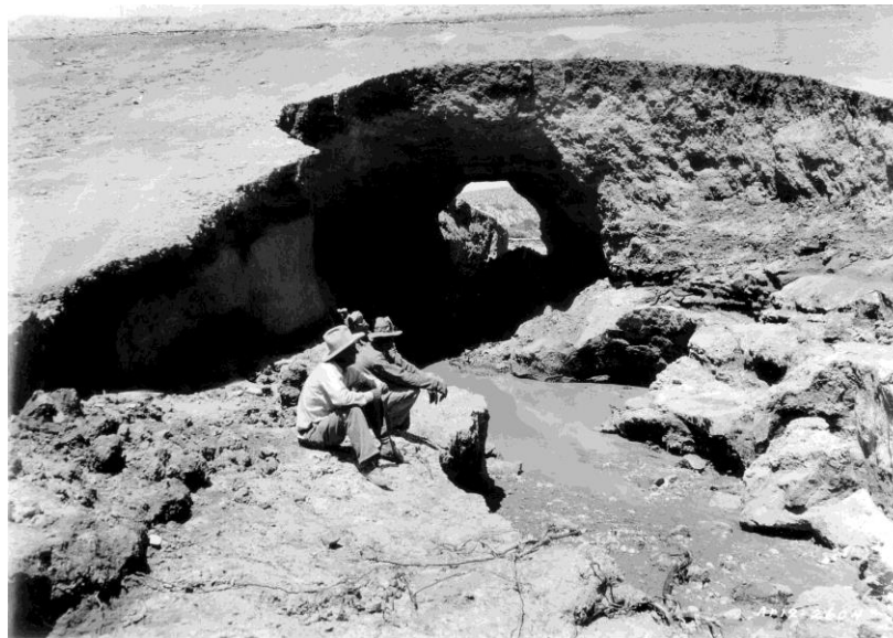
Figure 1.15 The May 1937 piping failure of a dam in Arizona (USA) comprised of dispersive soil (Image source: USDA NEH 633.13)
