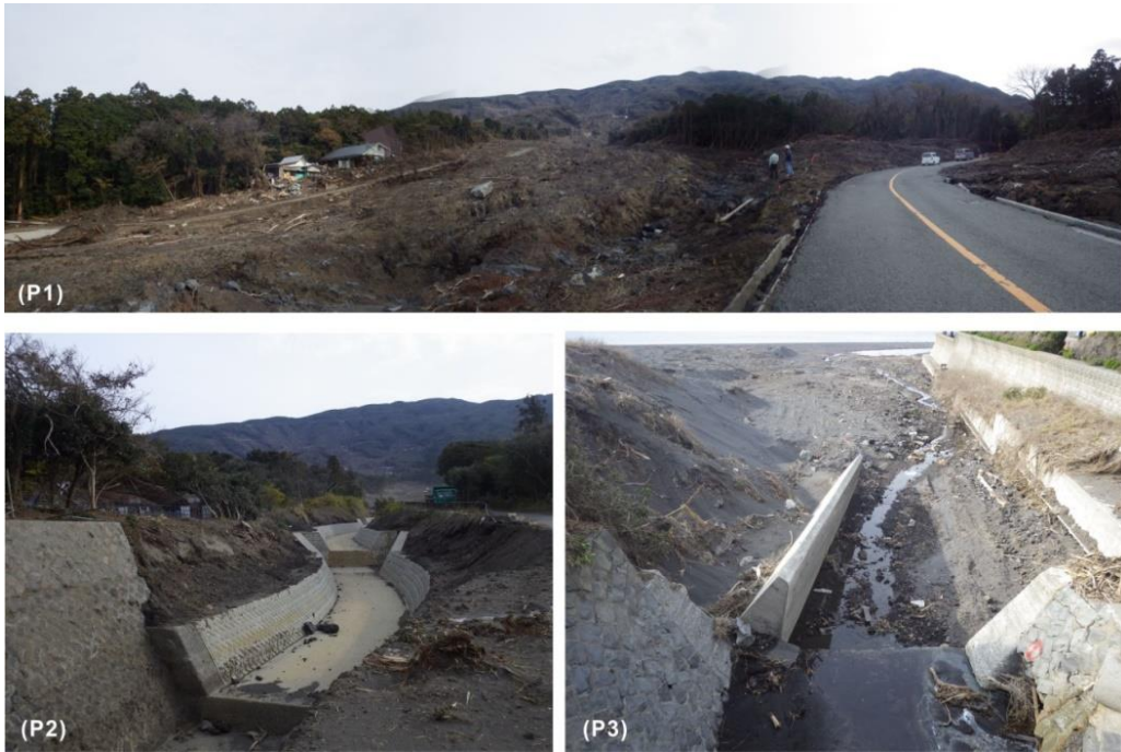
Fig. 5.8 Photographs after debris flows. The locations are marked on Fig. 5.7.
