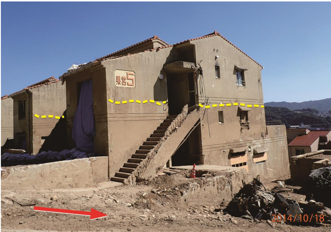
Fig. 6.8 The damaged prefectural housing at the pathway of the Midori-ga-oka debris flow. From the muddy trace on the wall, the flow depth of debris flow was about two-floors high.
